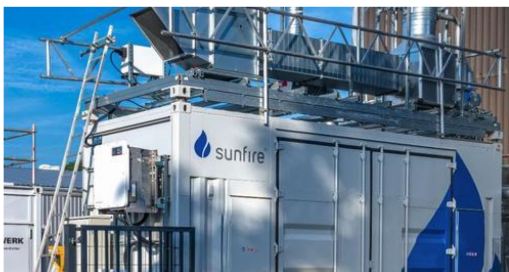
Fig. 1. 250kW electrolyser, Linden, Germany
